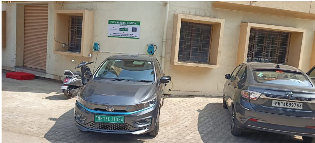
Setup of Electric Vehicle Charging Station
